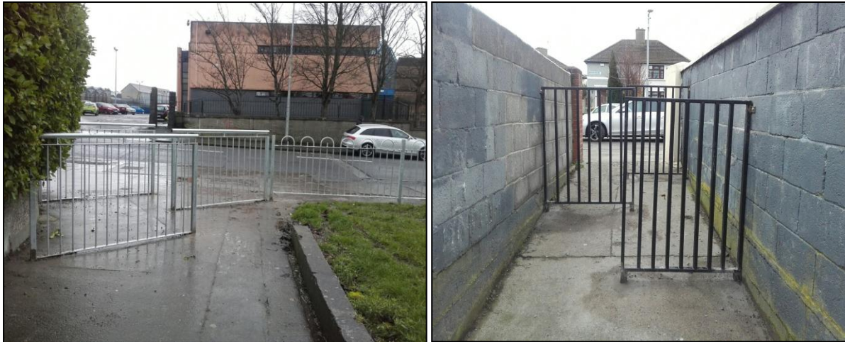
Barriers installed at Cardiffsbridge Road/Avenue and in the laneway between Ratoath Estate and Ventry Park
